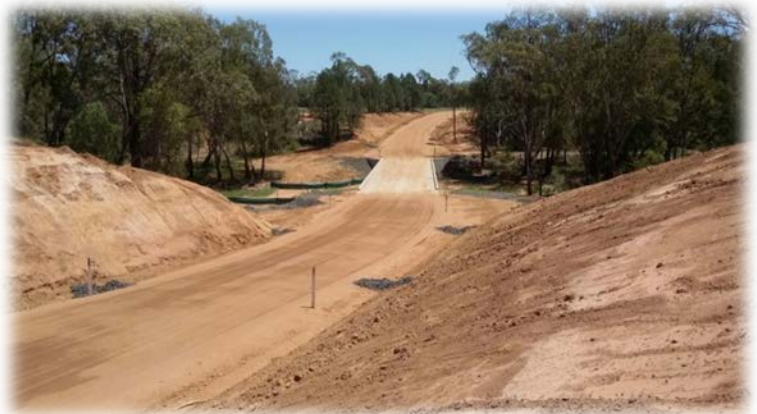
Photo on right: Replacement of the bridge on Wangmans Road over Baradine Creek near Kenebri was just one of five bridges replaced with loan funds under the timber bridge replacement program.
