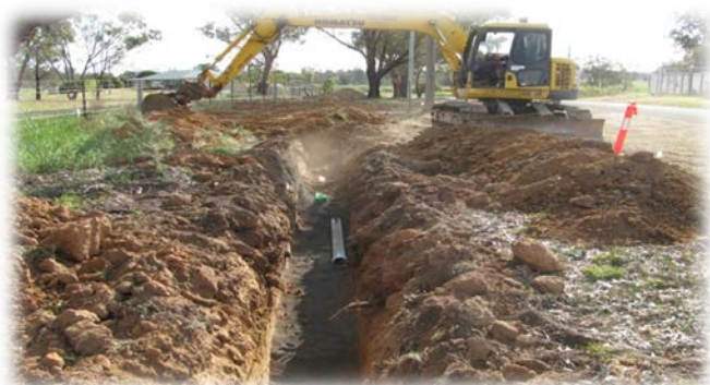
Installation of a new water main in Evans Street, Dunedoo. This work is being done under the water main extension programme which aims to improve reliability of water quality in the reticulation network
